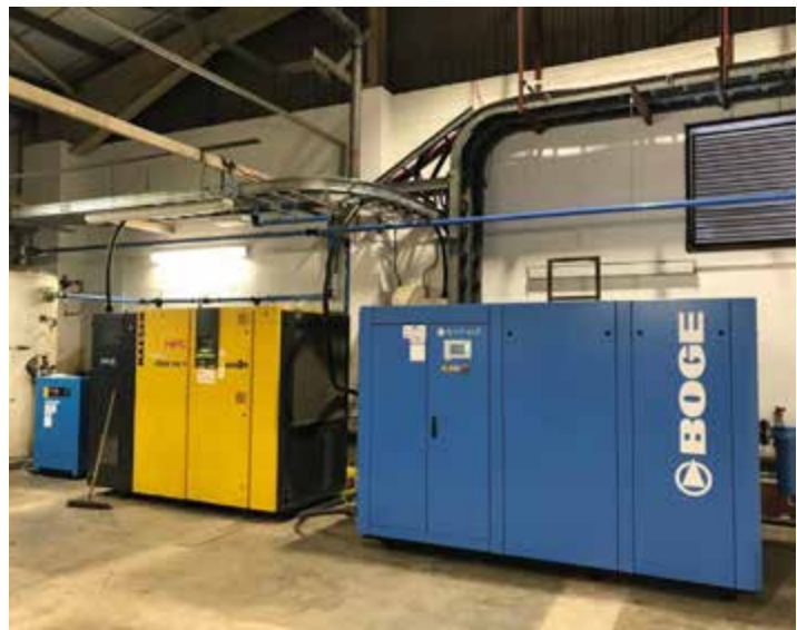
Compressor system upgrade with the installation of this Boge S111-4 LF Variable Speed Drive Compressor.
