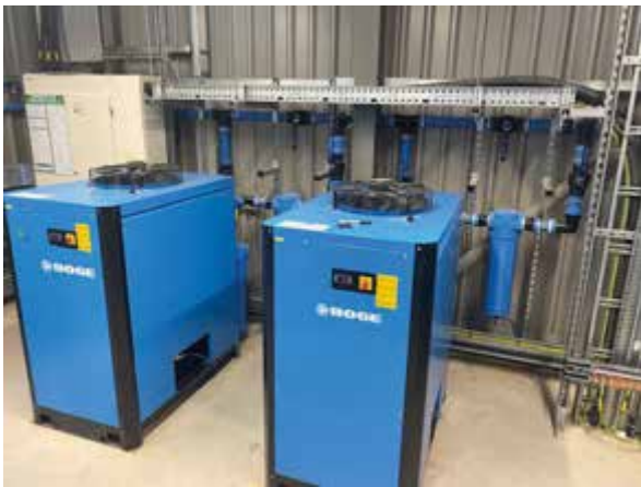
Twin 110kW, BOGE S111-4LF compressor package offering 100% duty back-up across the installation. The German built compressors will output 5.5-21.1 m 3 /min (194-745 cfm) @ 7.5bar. Also showing the duplex refrigerant dryer installation and full by-pass facility using EQO pipework system.
