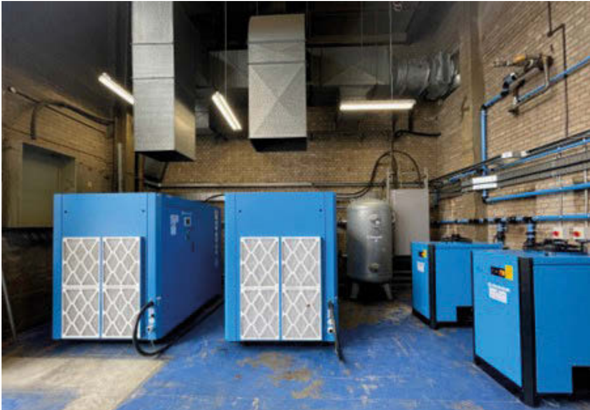
Twin 75kW, variable speed drive, Boge S76-4LF package with 100% duty back-up across the system. Both compressors are factory fitted with Duotherm heat recovery system for pre-heating water used in processes within the factory.
