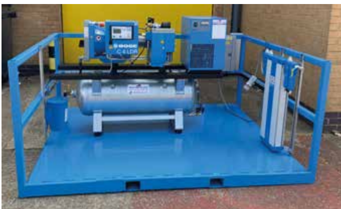
Bespoke compressed air package designed and constructed for our customer in the WCS workshop producing an air quality of ISO8573 Class 1,1,1. Utilising the Boge C4LDR Compressed Air Station with Walker Filtration Pro-dry and filtration package. All condensate treated by the Sterling CS75 oil/water separator.
